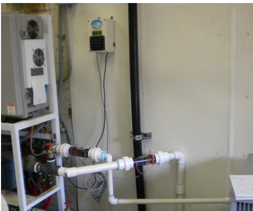
Existing bag filters may or may not be used, depending on existing water treatment.
